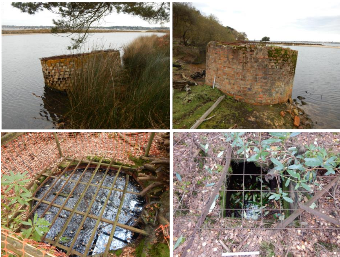
Figure 30 Photographs of the shafts at Seymers taken in 2017. Top left demonstrates the spalling on the bricks caused by the sea. Bottom left shows a circular ground level shaft and bottom right shows the timber lined square shaft.
